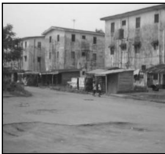
Fig. 4: Defaced buildings and housing neighborhood, dotted with makeshift (kiosk) extensions. At the foreground is a road already undergoing deterioration.
