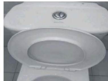
Fig. 3: Application of Double Flushing Cistern for Toilets in Masjid Wakaf Tembesu Kuala Terengganu
